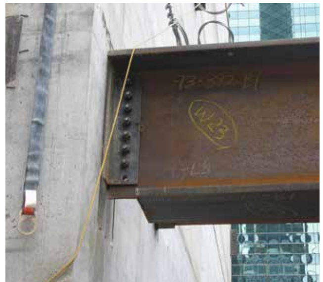
▼ Figure 2. Beam coped at the bottom flange.
